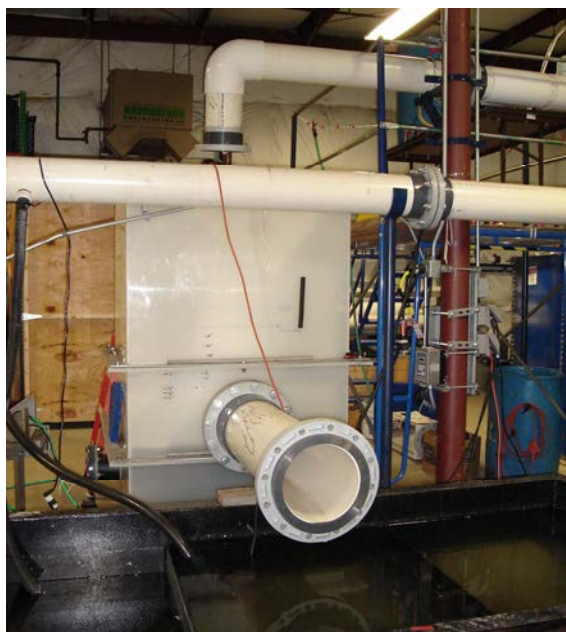
Figure A-2: View showing Up-Flo™ Filter overhead Inlet Pipe, Outlet Pipe and Collection Basin
