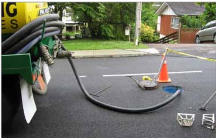
Fig.7 Sediment is removed from the sump with a vactor hose. Man entry is not required for this step.
