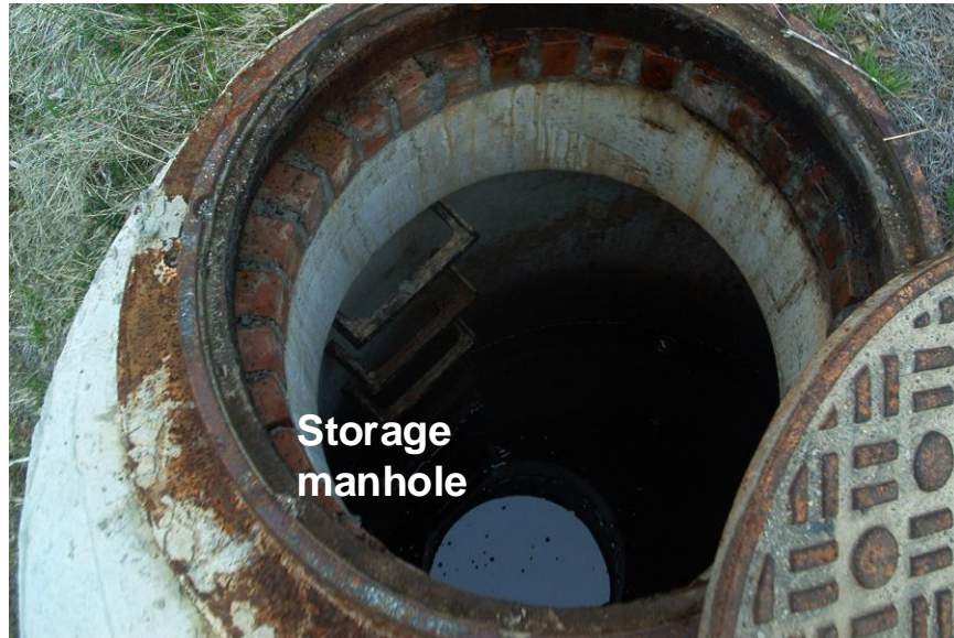
Figure 3: Storage manhole containing diesel fuel before pollutant removal:
