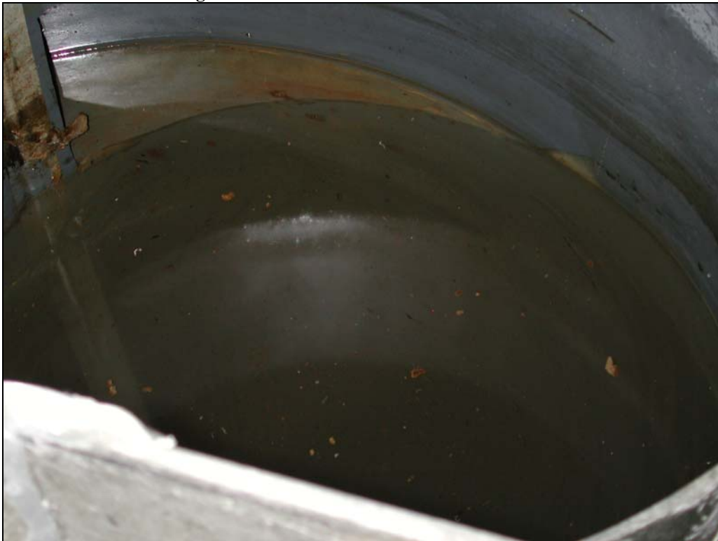
Figure 20. Inner chamber after 250 GPM test
