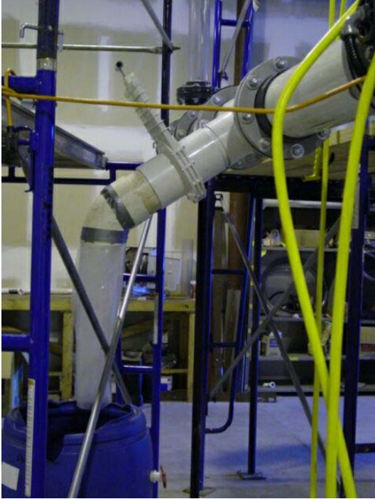
Influent Sample Valve (Gate)
