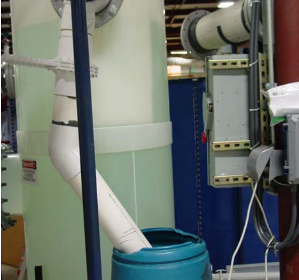
Influent Sample Valve (Gate)
