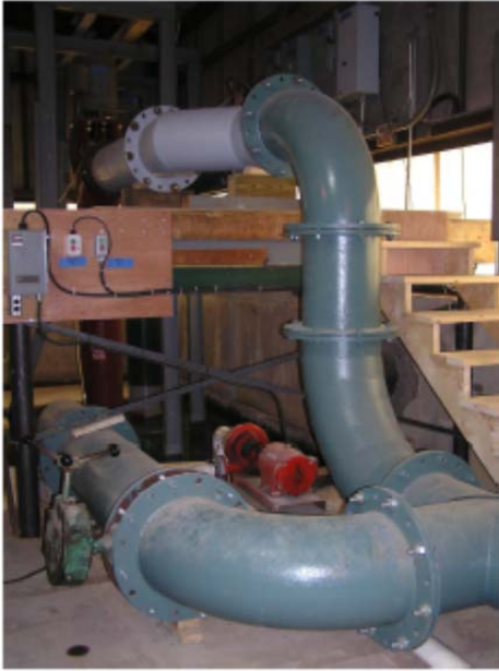
Figure 6: 50 HP and 20 HP Supply Pumps
