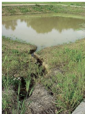
No Pretreatment: Without pretreatment, sediment can enter The main treatment cell and inlets can erode.
