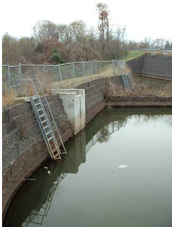
Maintenance Access and Safety: Steep side slopes make maintenance difficult and are a safety hazard.
