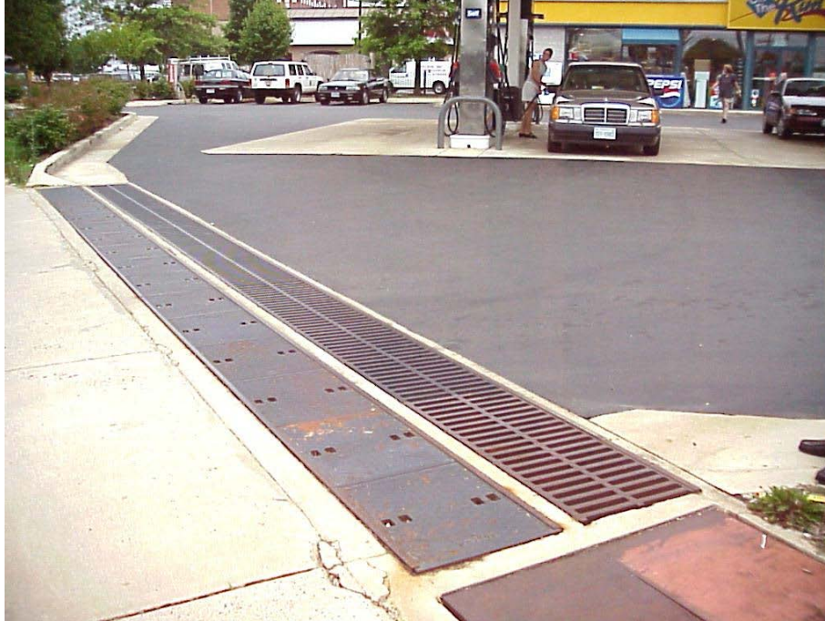
Figure 12.7. Perimeter Sand Filter
